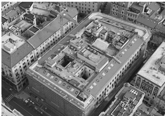
Hilton Doubletree – Trieste building. Pramac GGW200 generator set running on Natural-Gas is installed on the historic building's roof-top
